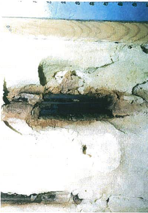
PHOTO 2—The 14 AWG test jig carried multiple runs at 120 percent level. After the 3rd and 4th runs, there was substantial charring of the insulation on the cable. When powered at 120 VAC, arcing immediately occurred on the damaged cable.
