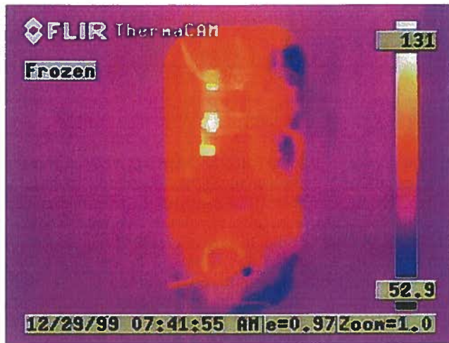
PHOTO 5—This thermal image shows the results of loosened connections on the thermostat and high limit switch of an electric water heater.
