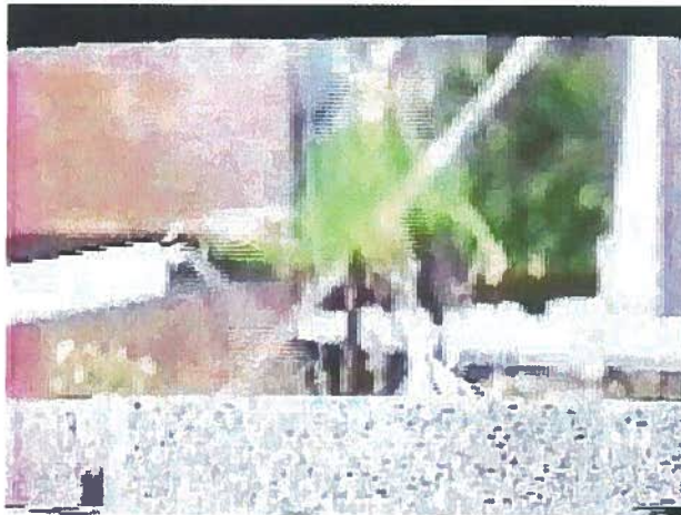
Photo 3 – Bonding Wire Failing When Carrying Lightning Current
