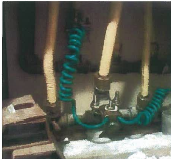
Photo 1, Showing 'Air Core' Inductors In Bonding Connection
