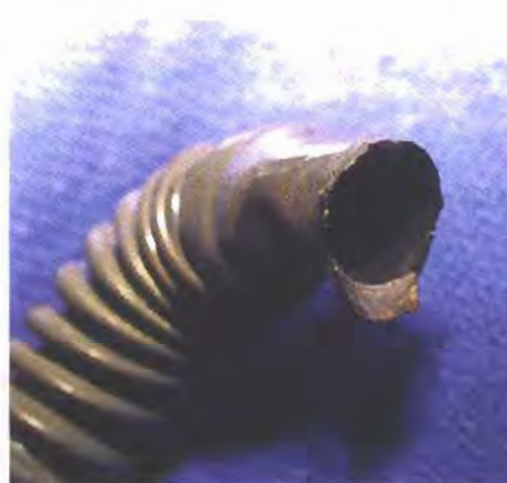
Photo 2. End of flexible gas line with most of the flare having melted due to electrical activity.
