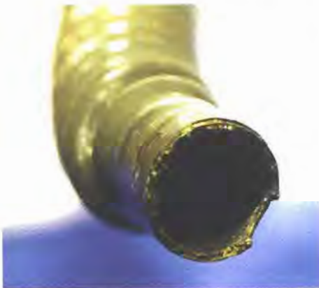
Photo 3. End of gas line with flare being destroyed by electrical activity.
