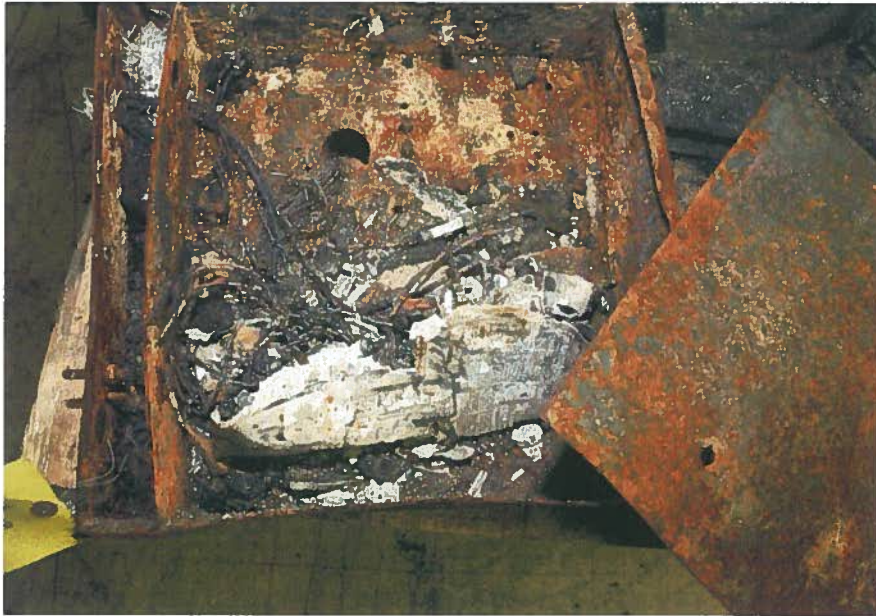
Photo 12 – Internal Parts Of Hot Tub Controls
