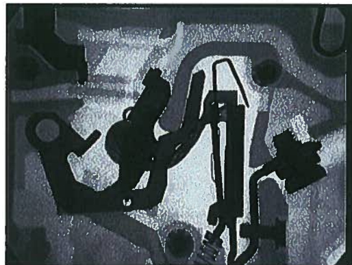
(Photo 9) An externally fire damaged breaker, with x-ray showing match to the library image of Photo 8
