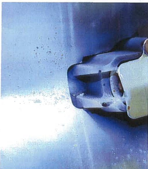
(PHOTO 4) —Shows a contact at the right end of a 300 watt fixture beginning to arc, spewing off molten copper.
