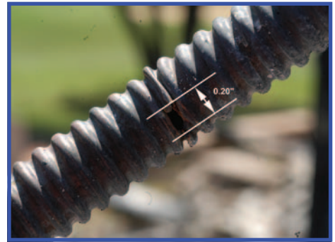
Figure 3: Perforated CSST pipe from fire in Edmond, Oklahoma.
