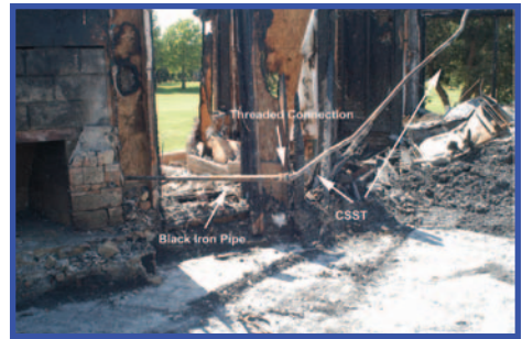
Figure 4: CSST tied to Black Iron pipe from fireplace.
