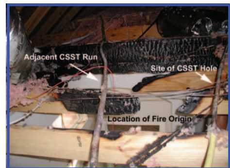
Figure 5: Attic fire during lightning storm Cedar Hill, Texas.
